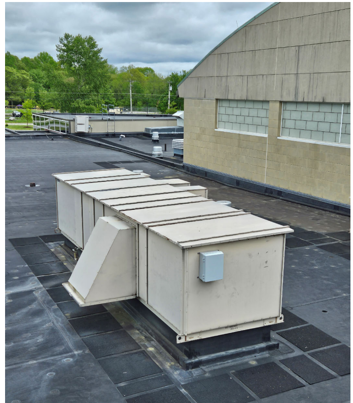
One of the school's RTUs (rooftop units)
