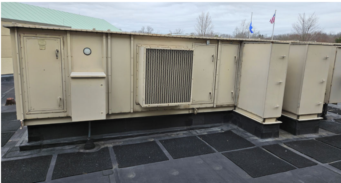
An AHU (air handling unit) at the east coast high school
