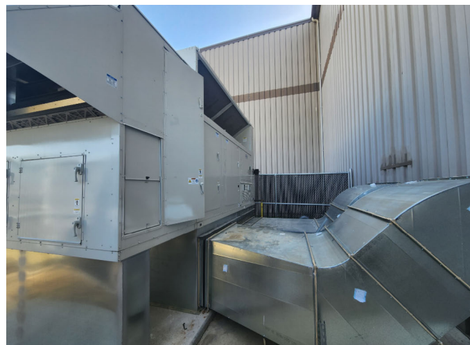
Restrictive duct geometry at the project site necessitated an innovative airflow measurement solution.
