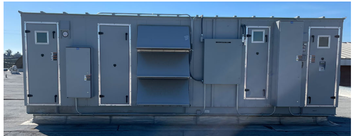
The versatile AFMS was easily installed in five retrofits (such as above) and one new unit (below).
