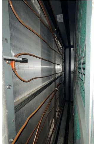
Outside, return, and mixed air (pictured) temperature sensors were installed.
