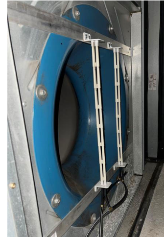
Airflow measurement probes were installed on the supply (pictured) and return fans.
