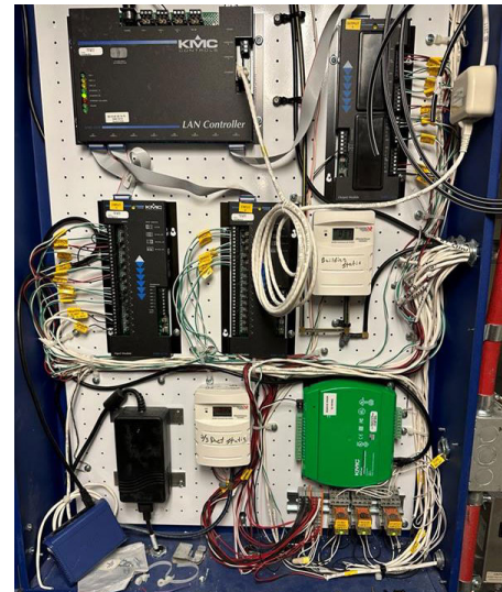
Data integration with the AFMS (green) was achieved through BACnet/IP over Ethernet.
