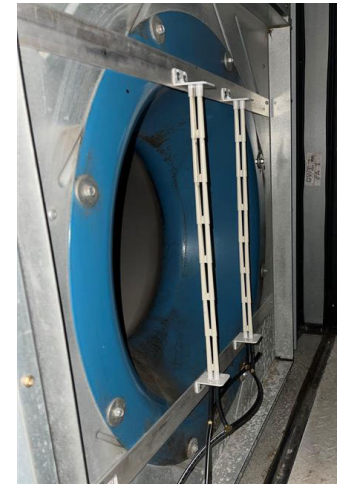
Airflow measurement probes were installed on the supply (pictured) and return fans.
