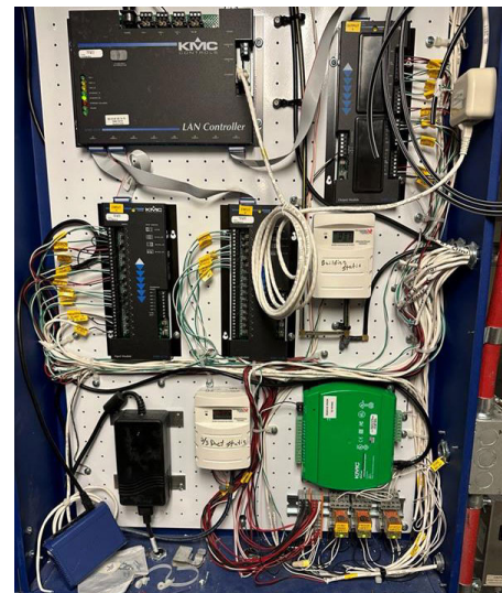
Data integration with the AFMS (green) was achieved through BACnet/IP over Ethernet.
